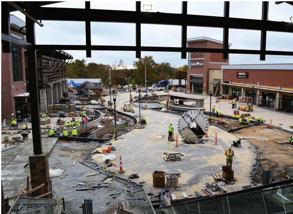
General contractors can subcontract landscaping companies when working on large projects. Photo: Ruppert Landscape
